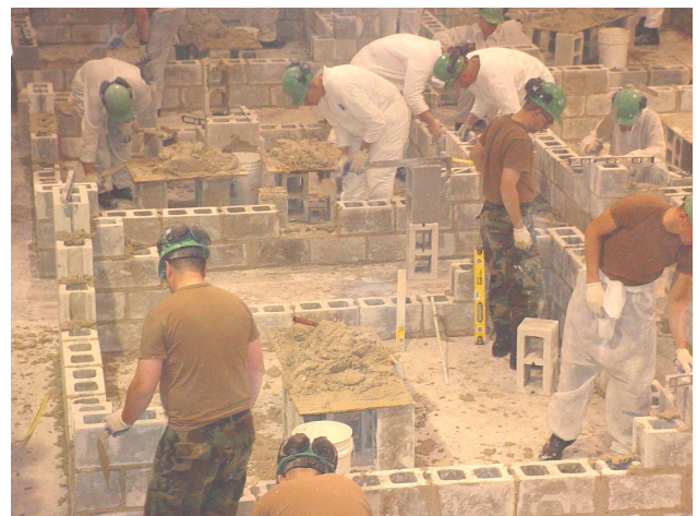
Carpentry students practice placement of concrete masonry units as part of the 21W10 MOSQ course.
