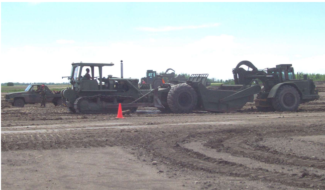
D-7 dozer and scraper in action at the Camp Grafton Local Training Area as part of the 21J10 MOSQ course.
